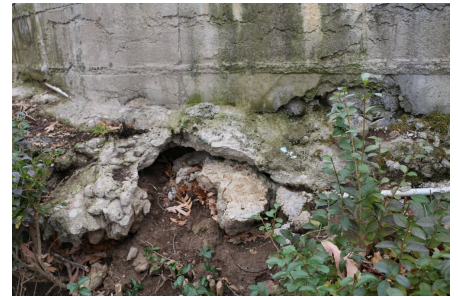
Cavity Beneath Wall
